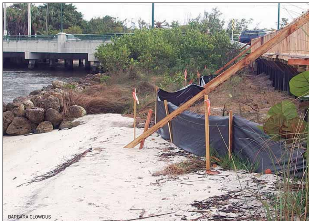
The Tech Center, formerly Dutcher's Cove, a project approved in 2008, started constructing a retaining wall that will hold fill to support the weight of a three-story building. In the foreground is the Pitchford's Landing property, which was not permitted to construct a seawall due to resident protests.
